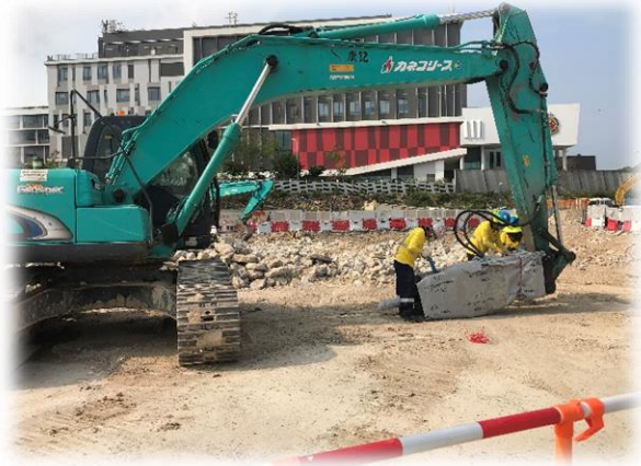
The breaker tips are wrapped with sound insulating material to reduce the noise
